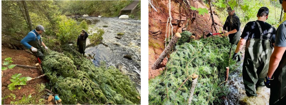
Building a balsam fir brush mat at the bottom of Leard's Pond spillway.
